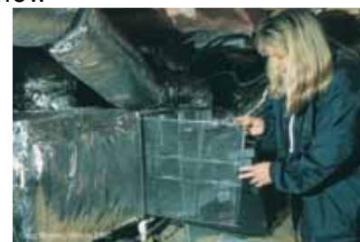
You should check your entire HVAC system each year, including your ductwork, to make sure air leaks are kept to a minimum.
