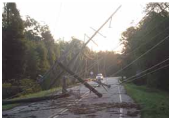
Damage such as this was not uncommon from Hurricane Irene. This triple circuit pole was broke by a tree on Davistown-Mercer Rd.
