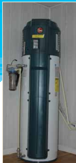
This Rheem heat pump water heater has proven to be approximately 138% more efficient than the previous 50-gallon conventional electric water heater that was in service before.
